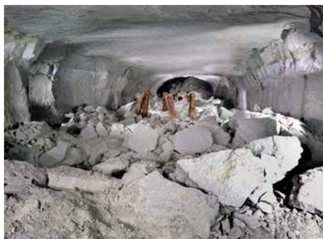
The development of the galleries at Marden relative to rock joints left mine ceilings very liable to collapse. Note the pit props which have failed to support the ceiling
